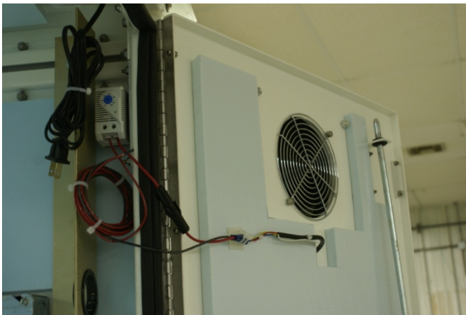
INSIDE VIEW OF EXHAUST FAN WITH DOOR OPEN
