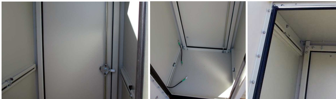
Internal views of Type 4 enclosure
